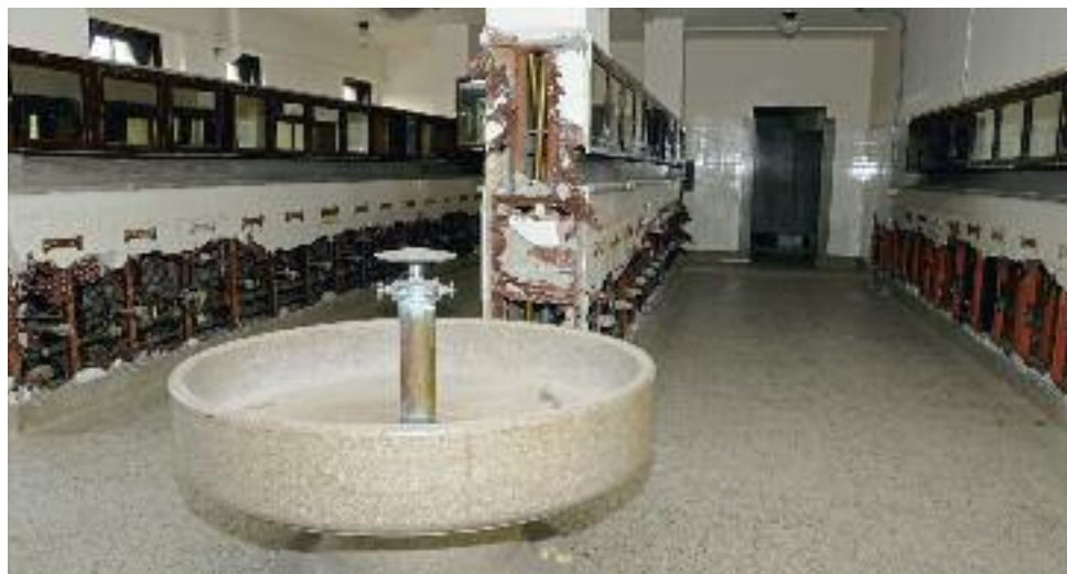
Rows of sinks have been removed from the communal bathrooms on the third and fourth floors of Newman Hall as renovations get under way in the School.
