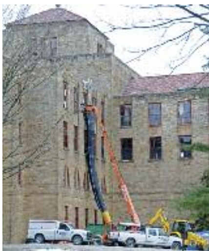
By mid-December, demolition work was under way in St. Bede and Newman halls.
